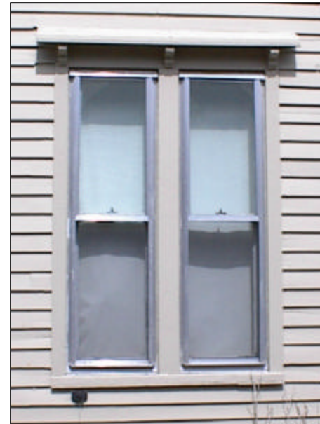
Upper Left: Paired windows with a simple decorative hood supported by small brackets is a common Italianate detail.
