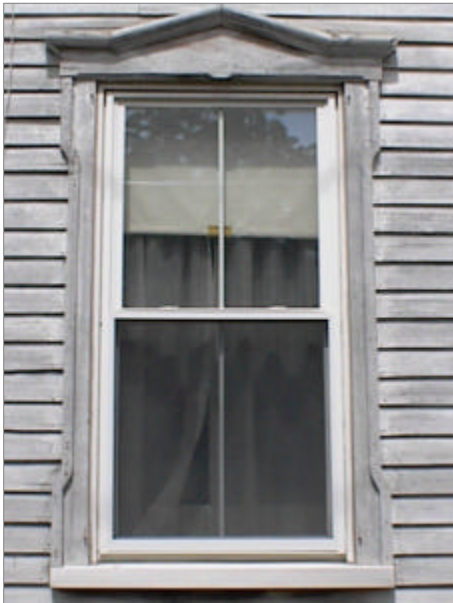
Above: Decorative trim (surrounds) around the window is an important character-defining feature to maintain whether or not the sash needs to be replaced.
